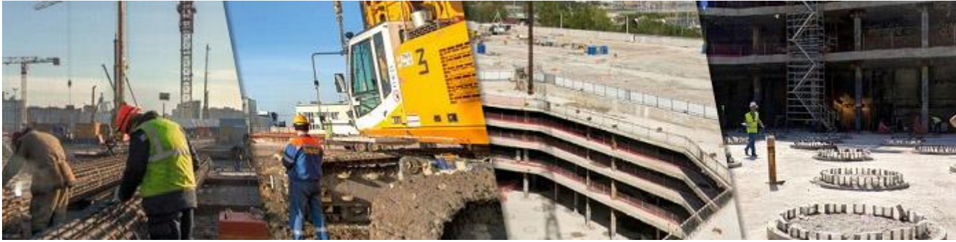
Four spherical panoramas show the most interesting places on the zero cycle of construction site work.
